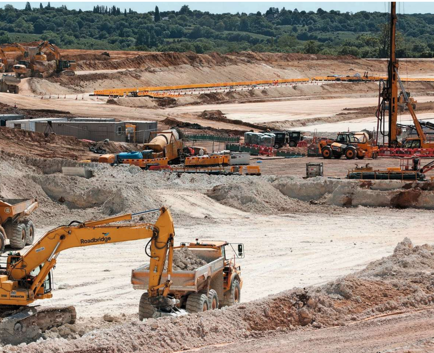
Construction is under way at the HS2 South Portal site in June 2020. This is the launch point for the two Chiltern Tunnel TBMs (tunnel boring machines). Next to the M25, the South Portal site is the largest construction site on Phase 1 and HQ for the main works contractor - Align JV. Nick Smallwood says that the industry can learn from projects such as HS2 because on such a large project, it would be impractical to leave it entirely with Network Rail. HS2 LTD.
