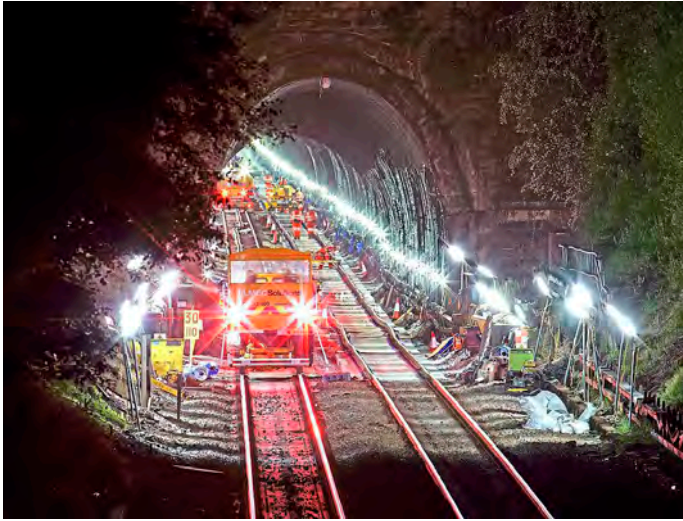
Engineering work takes place in Clay Cross Tunnel (Derbyshire) on May 29. The rail sector suffers from an ageing workforce with some 50,000 workers expected to retire by the end of the decade. MICK TINDALL.
