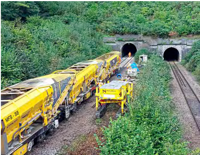
Track renewal and re-ballasting takes place at the Southern end of Dinmore Tunnel (Herefordshire) on September 18. Safety must remain the primary concern when NR chooses how to prioritise maintenance spending in CP7. JOHN EDEN.
