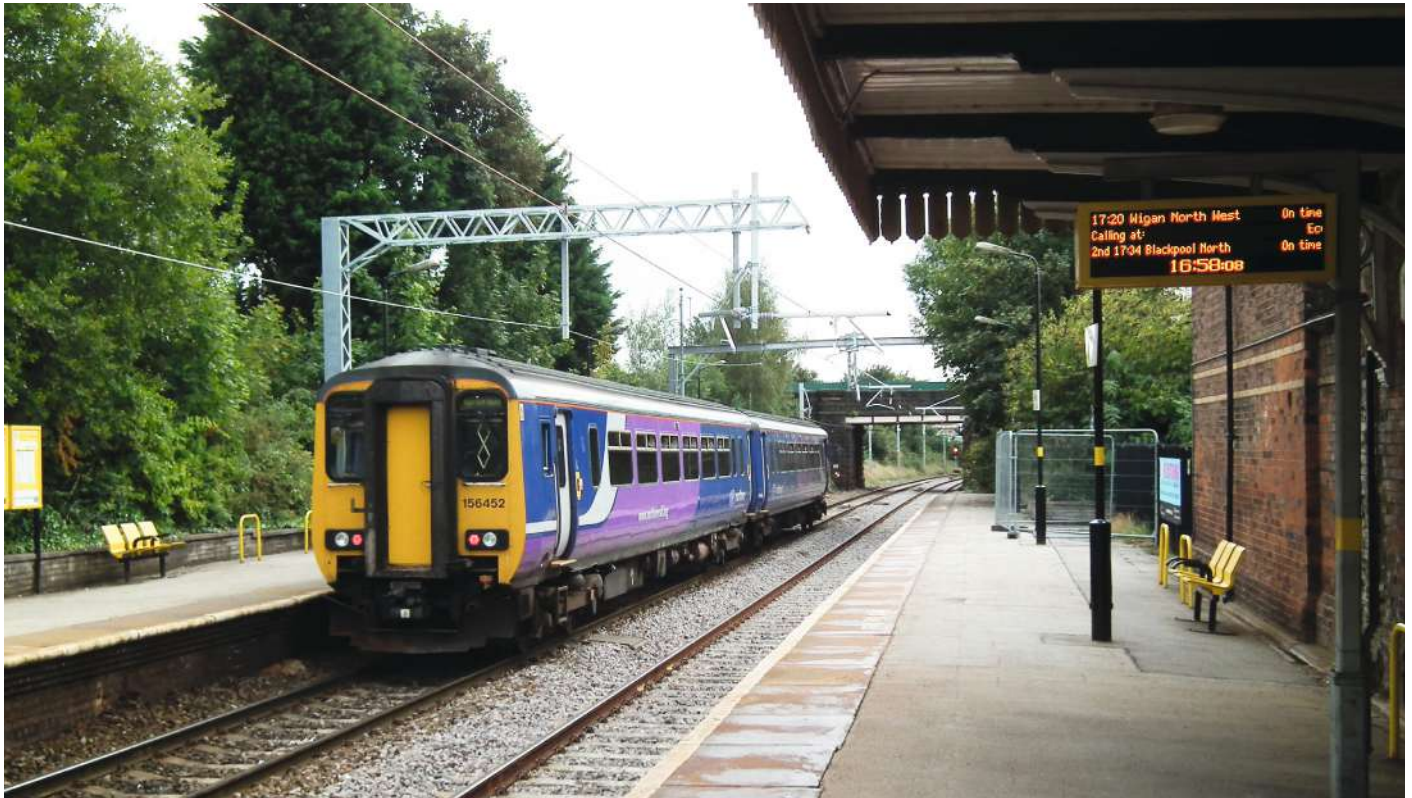
Prescott station on the Liverpool-St Helens-Wigan line on August 27. Electrification on this route is at an advanced stage, and catenary installation at Prescott station is complete. Ian Prosser is concerned that Network Rail's standards on the North West electrification project are inadequate. MIKE HADDON.
